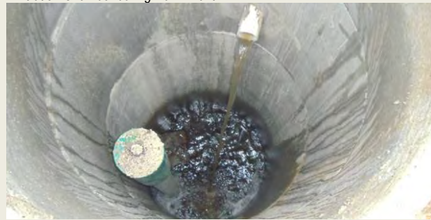
Infiltration Chamber during Rain Event
