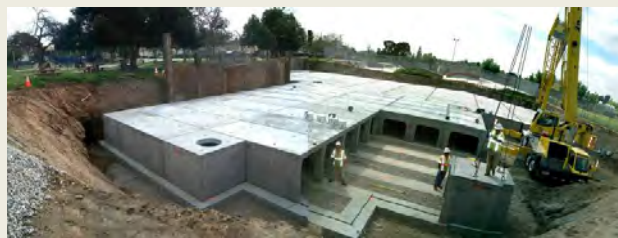
Underground infiltration gallery in Garvanza Park
